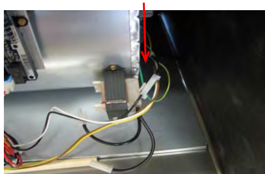
L1 harness connected to blower motor
